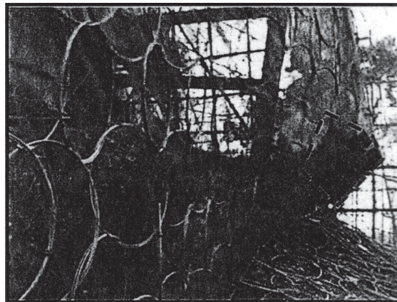
Figure 8. A photo showing the deflected shape of the rockfall fence. The boulder is highlighted by dotted lines
